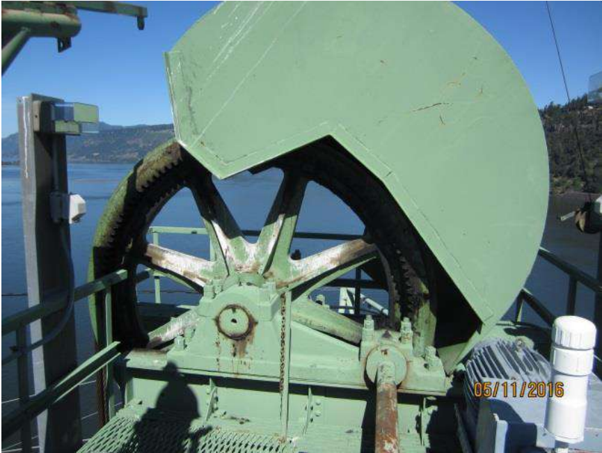
Figure 2: General view of rack and rack pinion.
