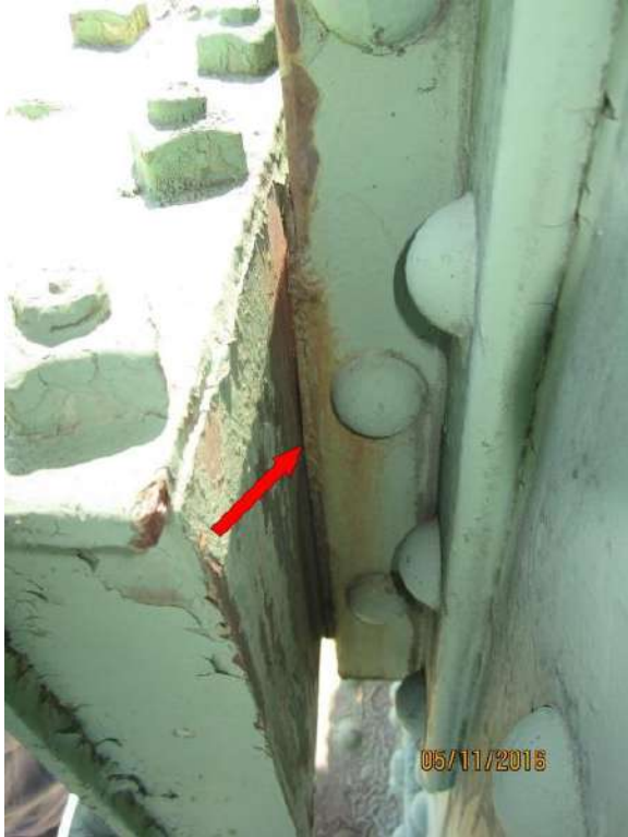
Figure 11: Northeast lower span guide. Note the addition of a wedge shaped shim
