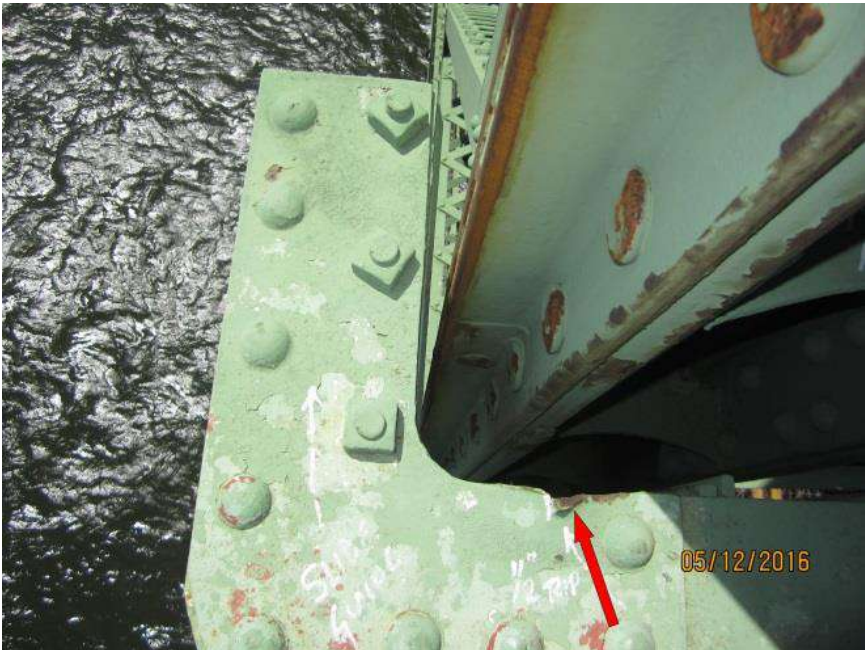
Figure 8: Southeast upper span guide. Note damage in longitudinal direction due to over-skew condition (arrow).
