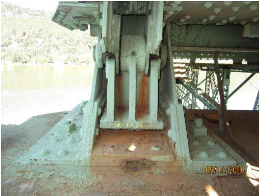
Figure 10: Northwest live load support. Note evidence of contact with the fixed structure at the left side of the rocker.
