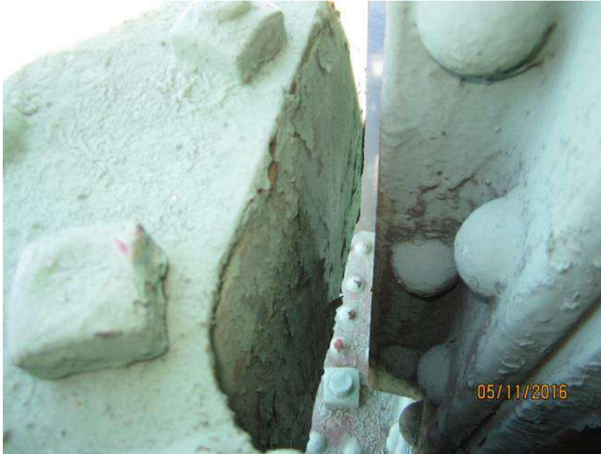
Figure 9: Northwest lower span guide. The span guide is not in contact with the guide rail.
