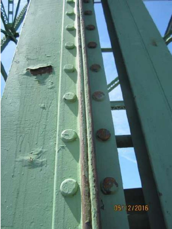
Figure 6: Southeast span guide rail. Note damage to rivets that secure the guide rail to the structure at the right side of the guide rail but no damage to the guide rail.
