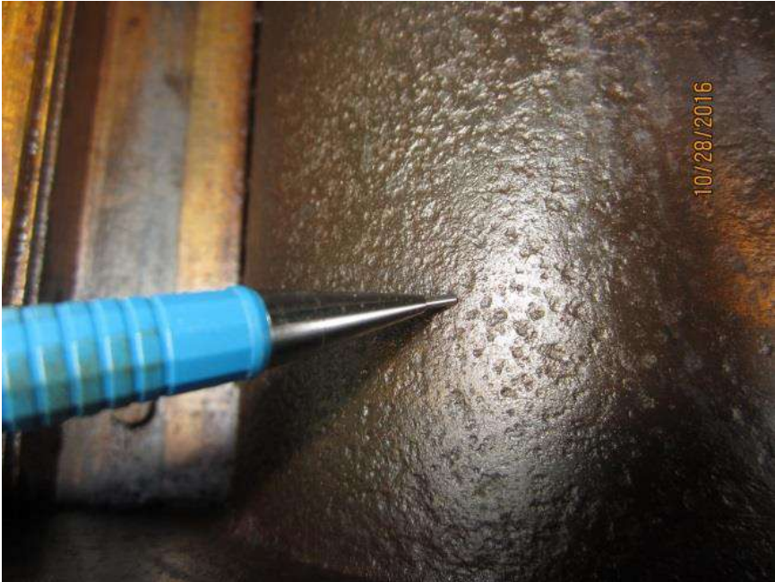
Figure 18: Southwest rack pinion bearing. Note the corrosion and heavy pitting on the journal.
