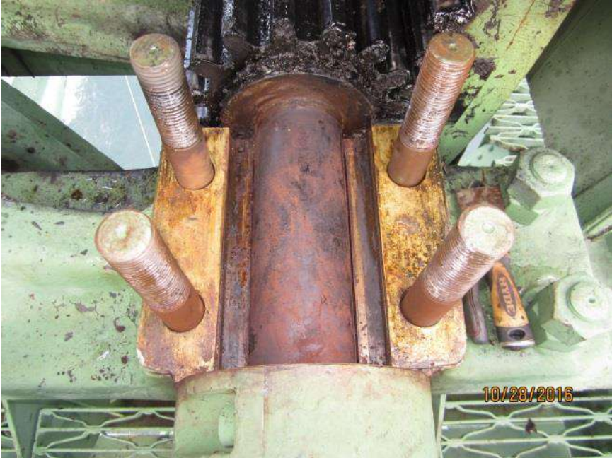
Figure 17: Northwest rack pinion bearing. There was no evidence of recent lubrication.
