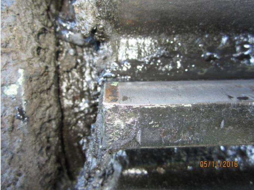
Figure 3: Rack pinion tooth cleaned for inspection.
