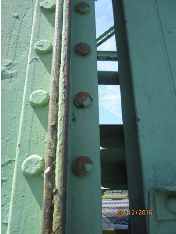
Figure 7: Close up of photo in Figure 6
