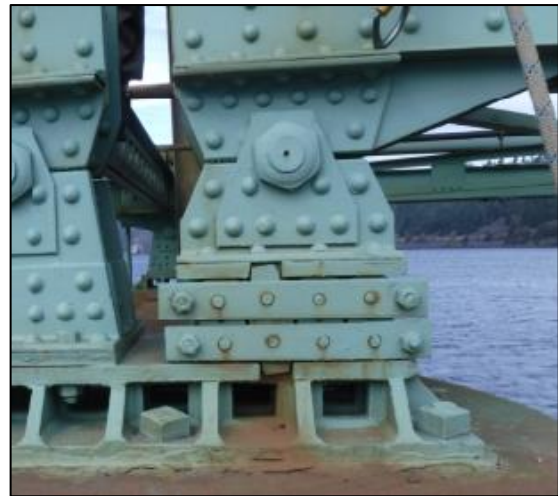
Figure 5 Pier 8 nested rocker bearing
