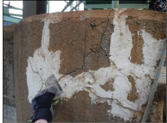
Figure 2 Existing epoxy paste
