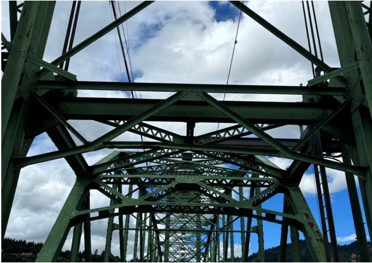
Figure: Damaged portal frame in the lift span (lower third of the picture)
