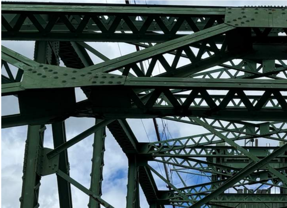
Figure: Damaged bottom chord
