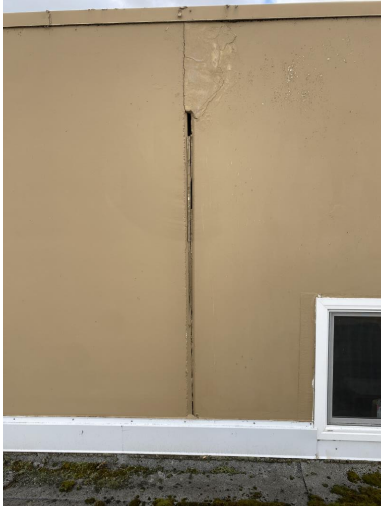
Photo 2: Crack patched across panel joint (not recommended) and missing/failed caulking
