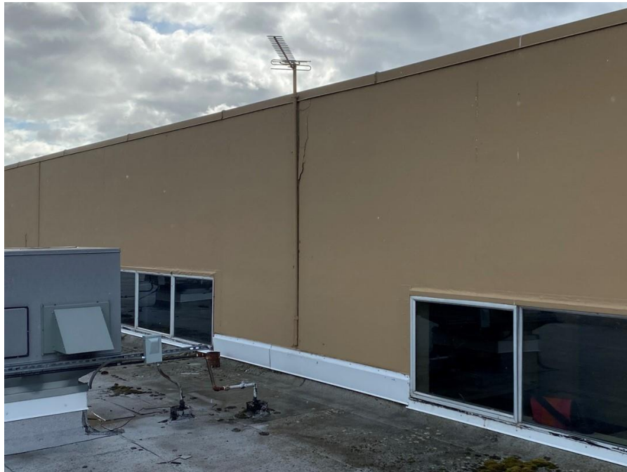
Photo 1: Typical cracking at panel joint
