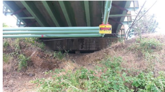
Figure 2. OR Abutment Erosion
