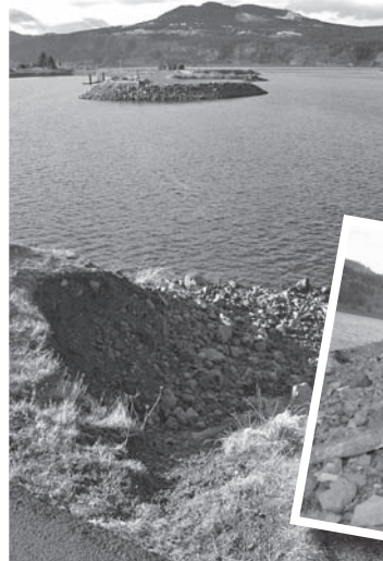
Rip-rap erosion below normal high-water level usually means a long wait for in-water work permits.
