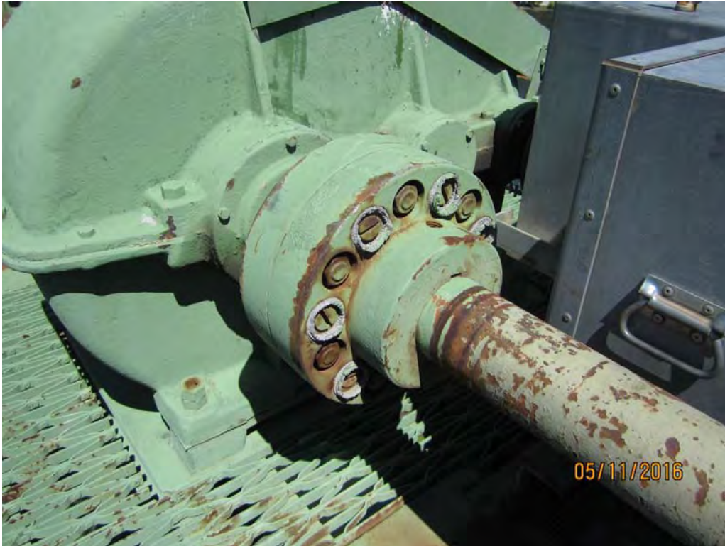
Photo 13 Rack Pinion Shaft Coupling. The coupling transmits torque via a bolt/pin installed with an elastomeric material through the coupling hubs. The elastomeric material is deformed and degraded.
