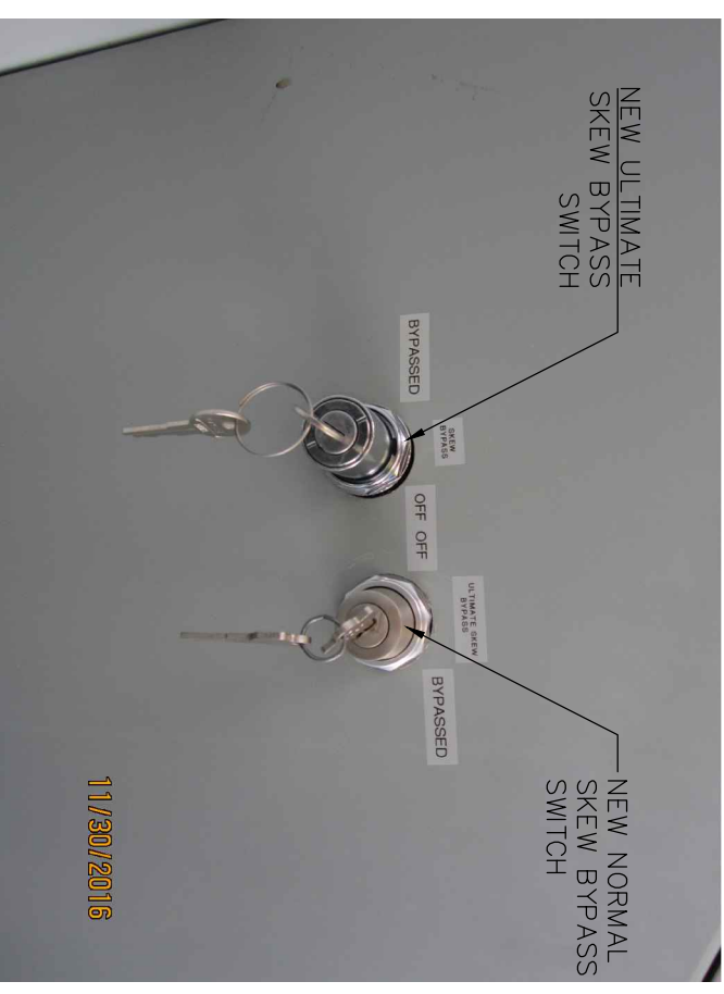
CONTROL CONSOLE (SIDE PANEL)
