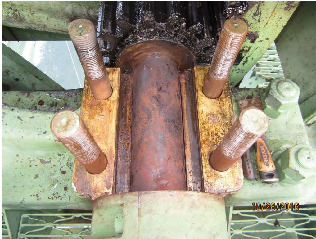
Photo 4 B1-NW Journal. View with bearing cap removed. The journal is in poor condition with heavy corrosion and minimal lubricant.
