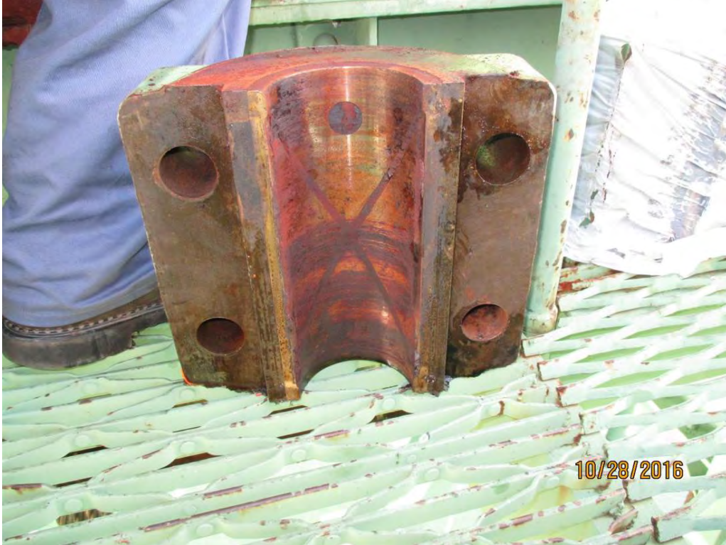
Photo 7 B1-SW Cap. View of cap prior to cleaning. Note the fretting corrosion and the clogged lubrication ports.
