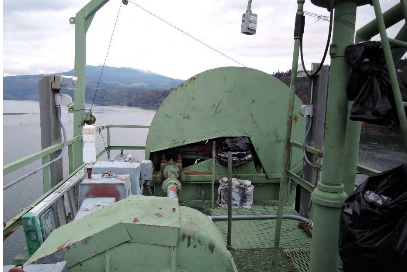
Figure 3. A sheave trunnion assembly in the north tower is shown beneath a partially open enclosure.
