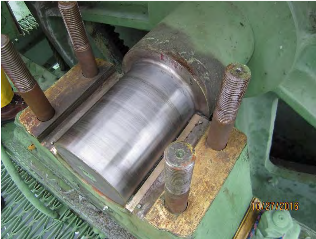
Photo 1 TB-NW-OB Journal. View with bearing cap removed and with the bridge in the seated position.
