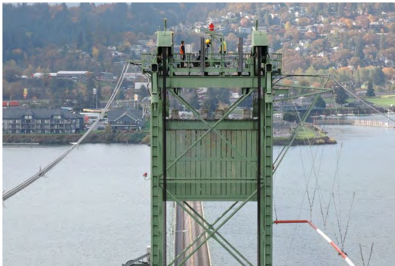
Figure 2. The south counterweight tower is shown with sheave trunnions and associated machinery.
