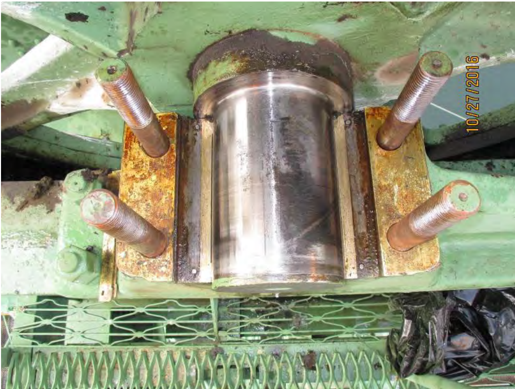
Photo 2 TB-NW-IB Journal. View with bearing cap removed and with the bridge raised for access to the portion of journal that is not visible with the bridge seated. Note the minor corrosion and dried lubricant.
