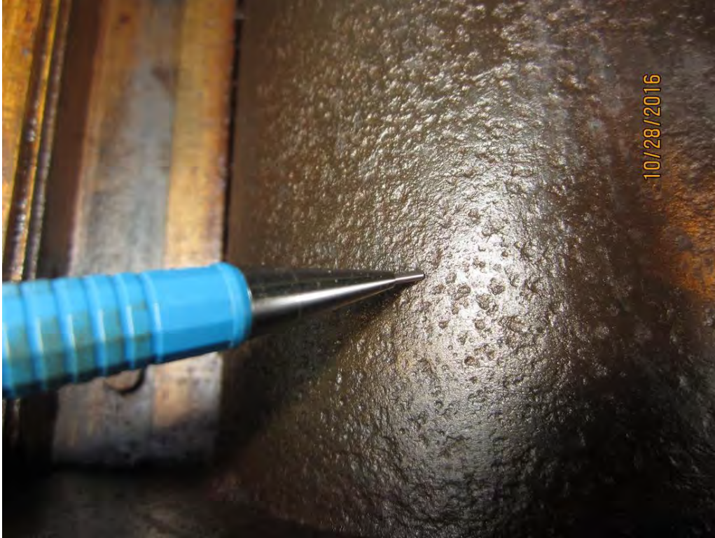
Photo 5 B1-NW Journal. Close-up view of Photo 4. Note the corrosive pitting on the journal.
