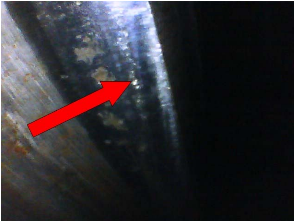
Photo 12 South Primary Reducer Gearing. Note the pitting (arrow).
