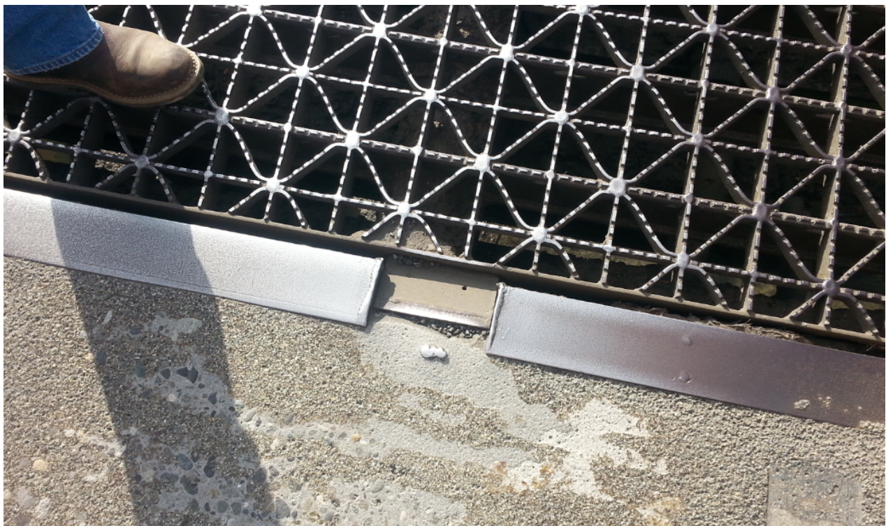
Broken steel header at Bent 20.
