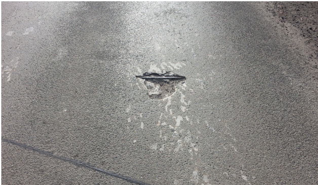
Pothole in Span 26, Joint at Bent 27.
