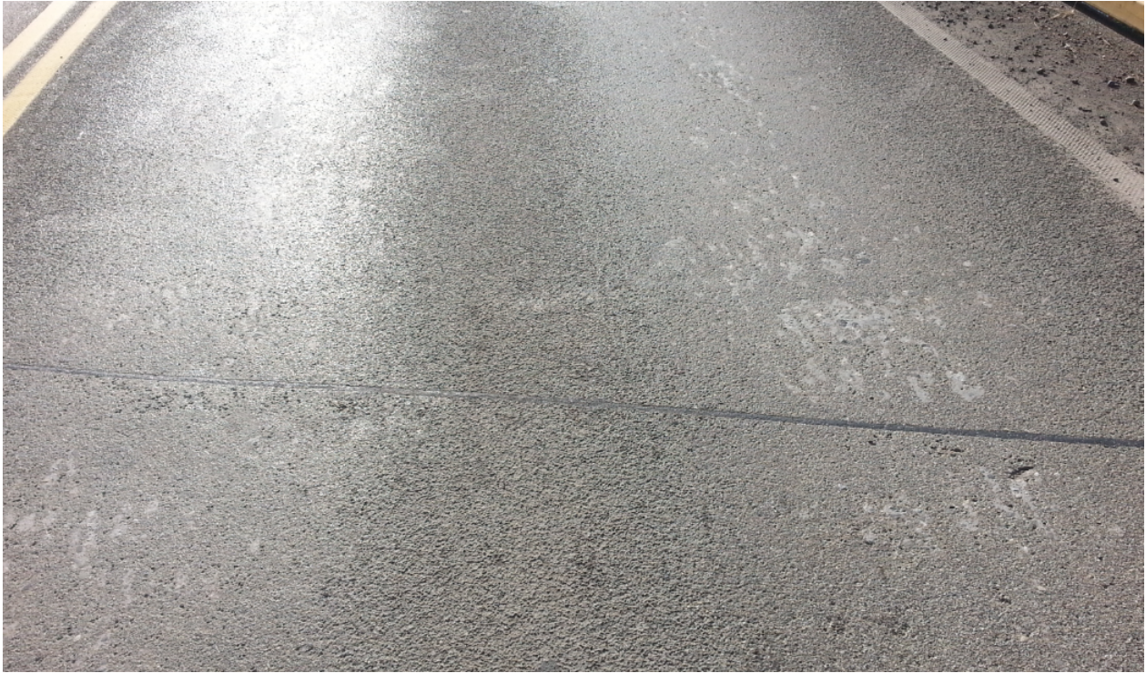
Worn overlay near Bent 25.
