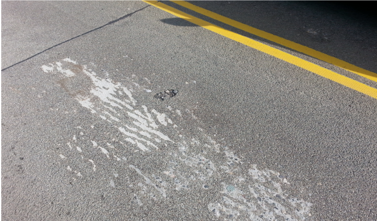
Worn overlay near Bent 22.
