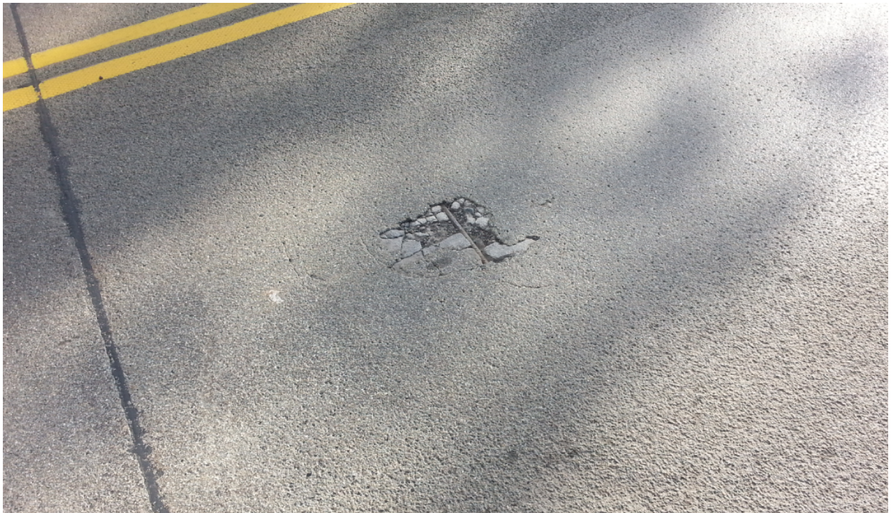
Pothole in Span 22, Joint at Bent 23.
