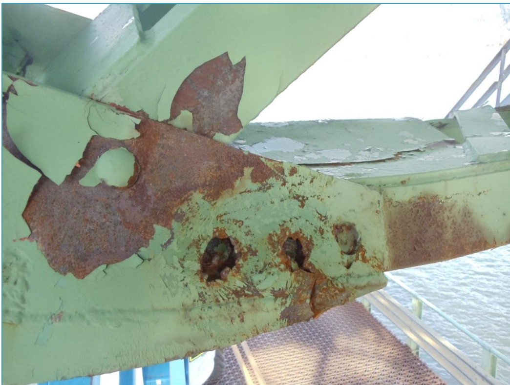
South face of fractured gusset at northernmost portal.
