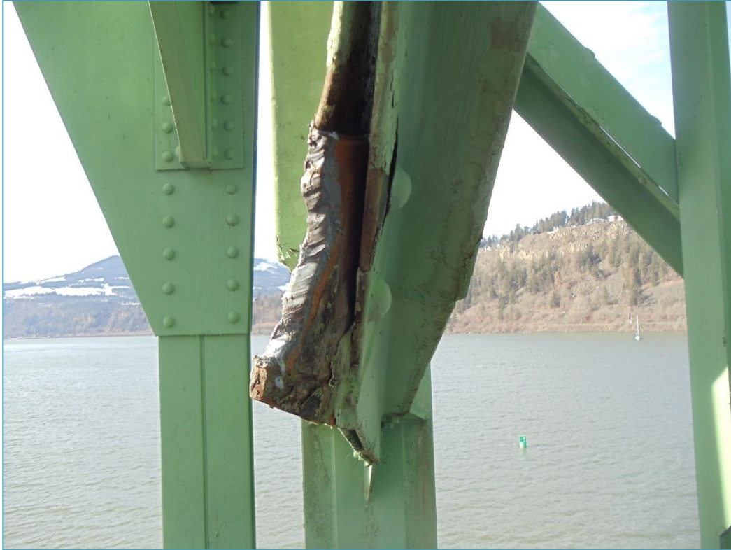
Bent/fractured gusset plate and buckled angles.
