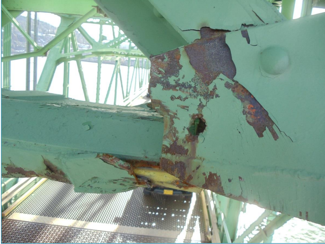
North face of fractured gusset at northernmost portal.
