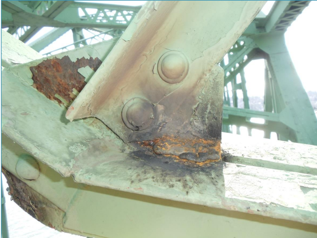
Field weld of fractured gusset plate.
