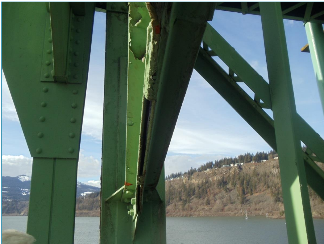
Buckled angles at vertical gusset plate at tower leg.
