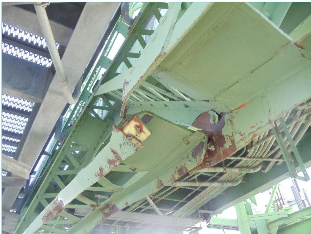
Portal damage at back face of tower.
