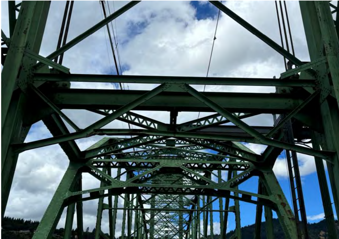
Figure: Damaged portal frame in the lift span (lower third of the picture)
