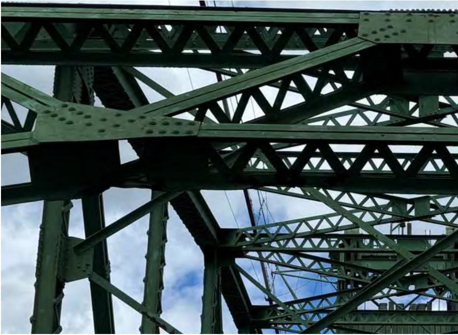
Figure: Damaged bottom chord
