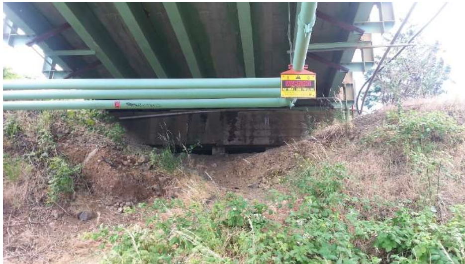
Figure 1. Erosion and Undermining at the South Abutment
