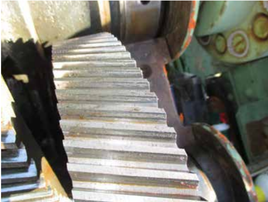
Photo 19. South Primary Reducer. View of east first reduction gear set, opening face of gear teeth. Note the pitting on the outboard (right) ends of the teeth.
