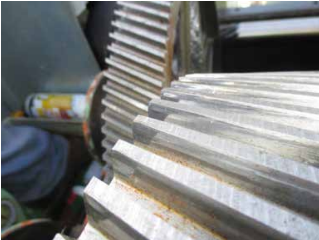
Photo 24. South Primary Reducer. View of east second reduction gear set, opening face of gear teeth. Closeup view of photo 23. Note heavier contact and light wear on the east (left) end of the teeth.
