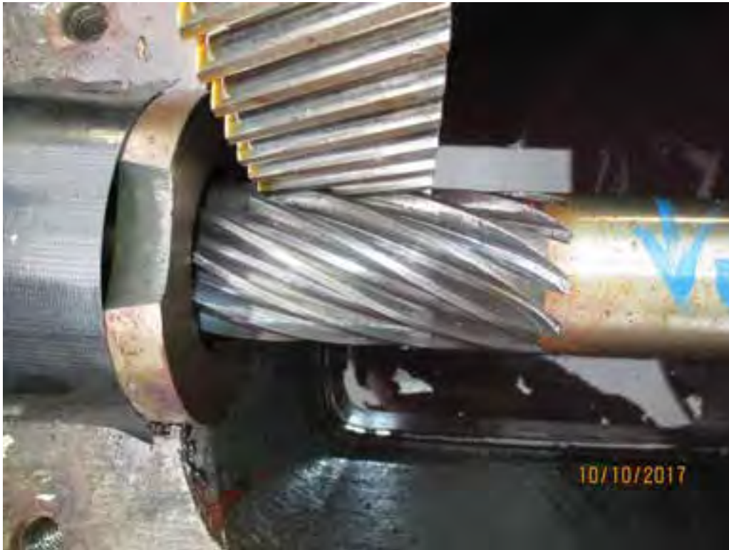
Photo 3. North Primary Reducer. View of east first reduction gear set.
