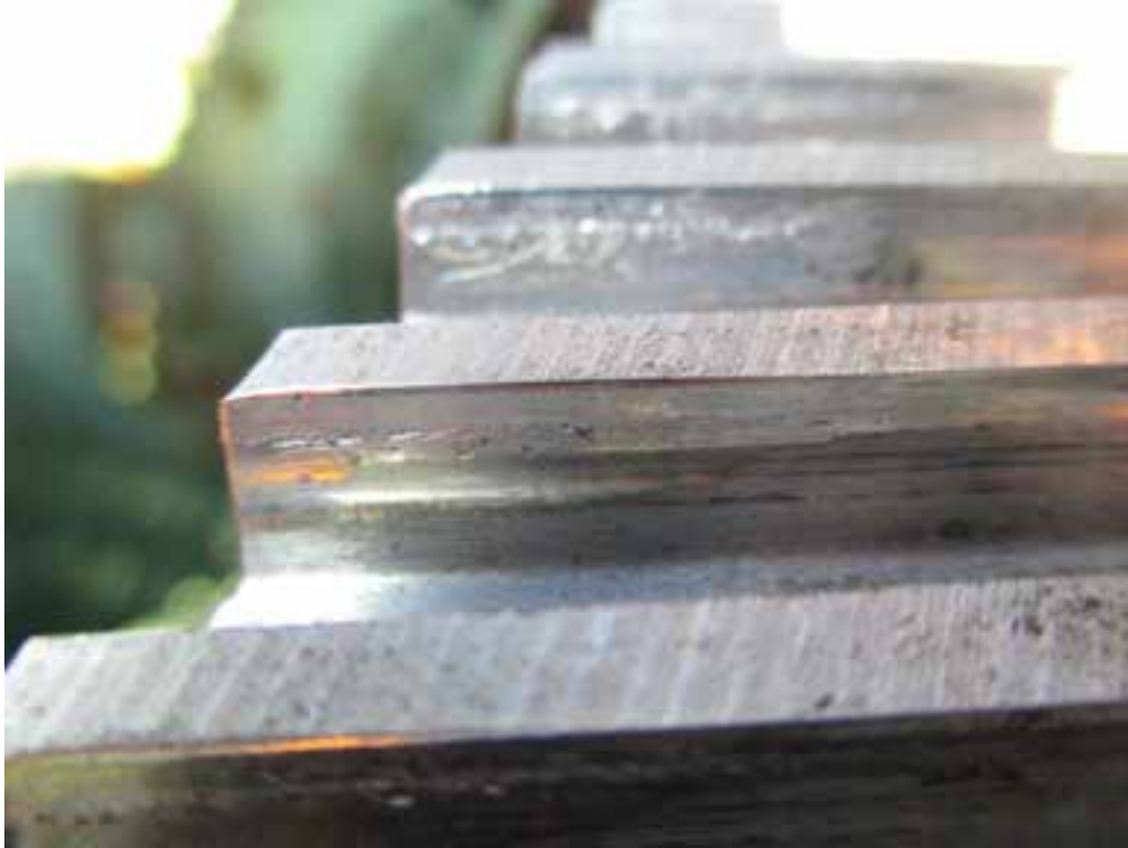
Photo 17. South Primary Reducer. View of west first reduction gear set, opening face of gear teeth. Closeup view of photo 16.
