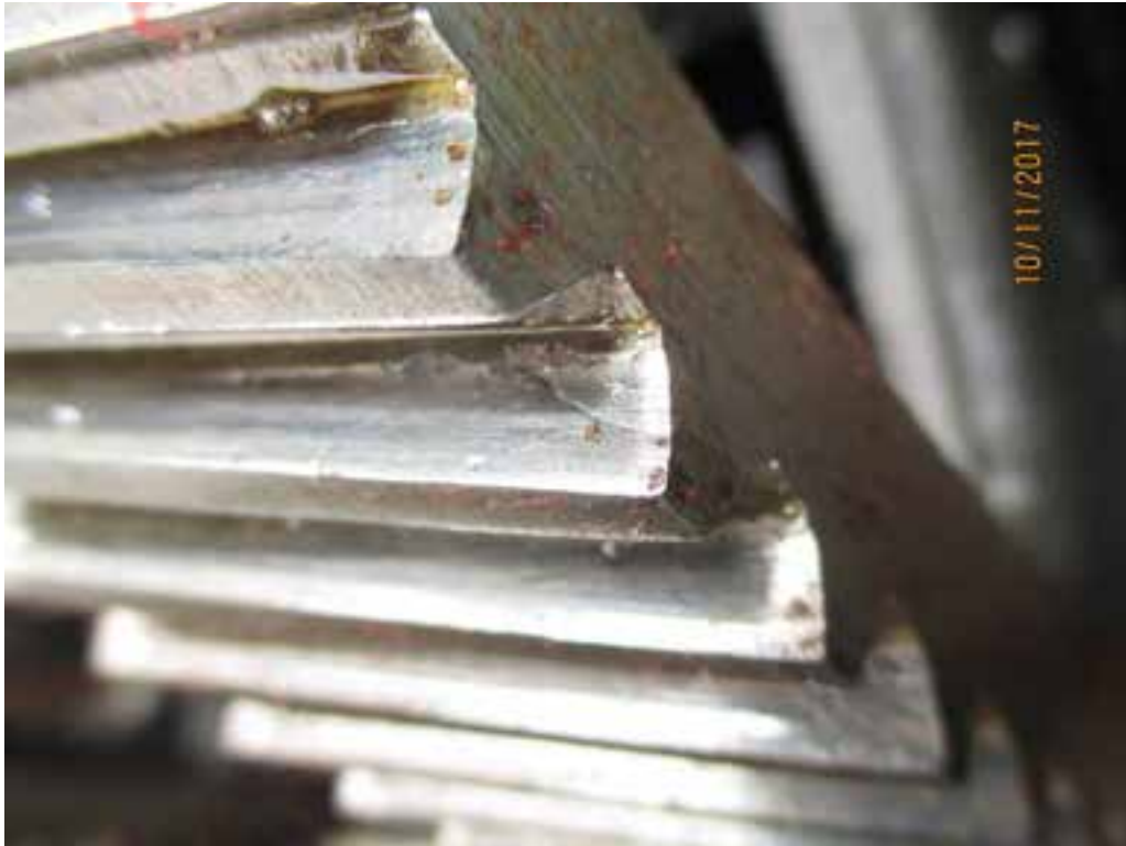
Photo 9. North Primary Reducer. View of west first reduction gear set, closing face of teeth. Note the damage on the west (right) ends of the teeth. Close-up of Photo 8. This damage appears to be the result of something passing through the mesh and not the result of an overload condition.
