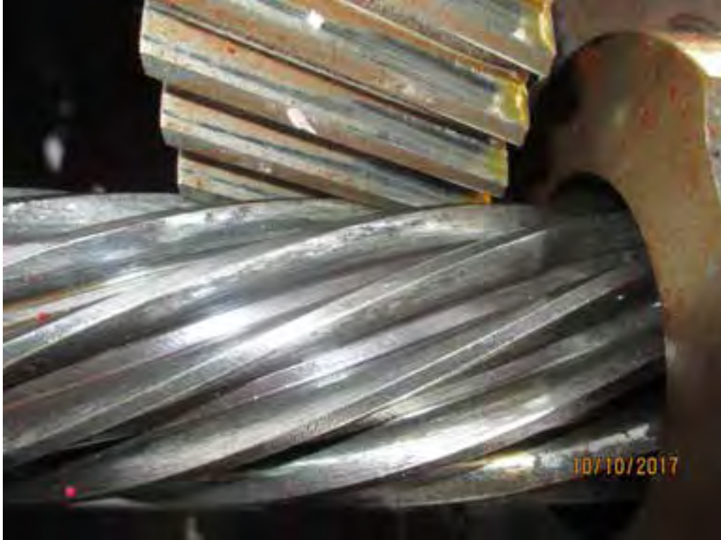
Photo 7. North Primary Reducer. View of west first reduction gear set. Note the heavier contact on the west (right) ends of the teeth.
