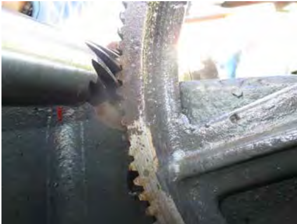
Photo 2. South Primary Reducer. View of the west high speed gear. The side of the gear rim and teeth are corroded.
