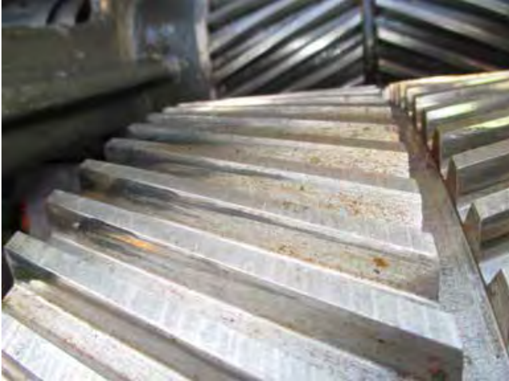
Photo 23. South Primary Reducer. View of east second reduction gear set, opening face of gear teeth. Note the contact and light wear.
