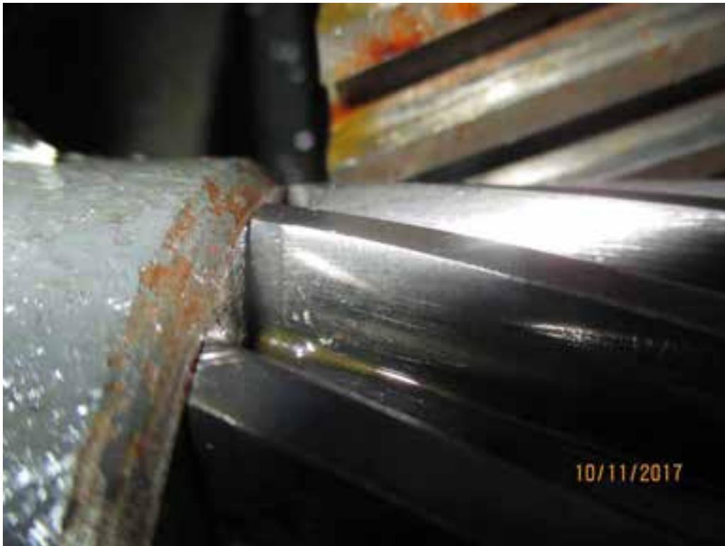
Photo 12. North Primary Reducer. View of east second reduction pinion, closing face. Small isolated pits were noted on the east (left) end of the teeth.
