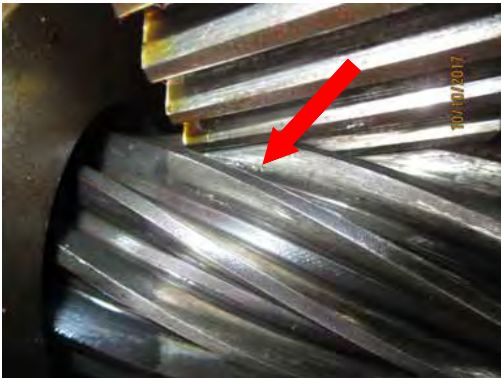
Photo 4. North Primary Reducer. View of east first reduction gear set, opening face of pinion teeth. Note the pitting (arrow) on the east (left) end of the teeth.
