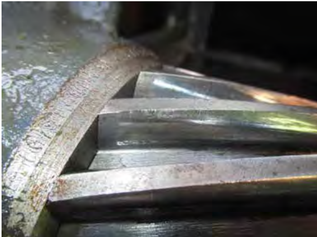
Photo 22. South Primary Reducer. View of east second reduction gear set, opening face of pinion teeth. Closeup view of photo 21. Note heavier contact and light wear on the east (left) end of the teeth.
