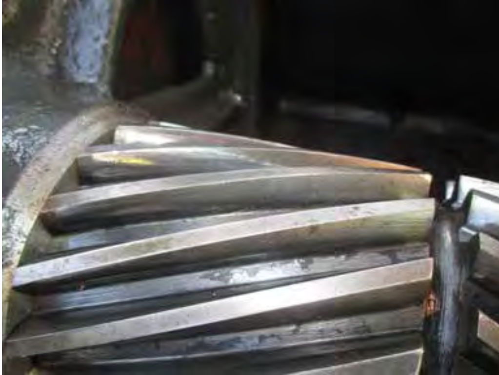
Photo 21. South Primary Reducer. View of east second reduction gear set, opening face of pinion teeth.
