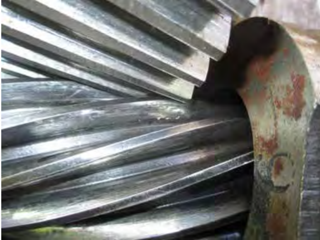
Photo 15. South Primary Reducer. View of east first reduction gear set, opening face of pinion teeth. Closeup view of photo 14.
