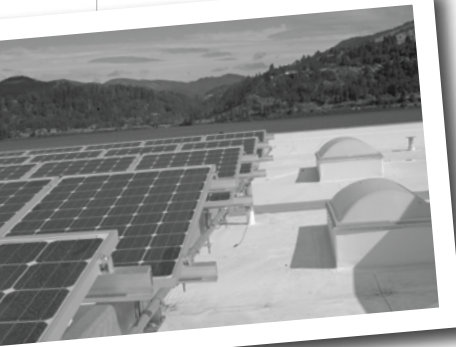
Solar Panels atop Halyard Building
