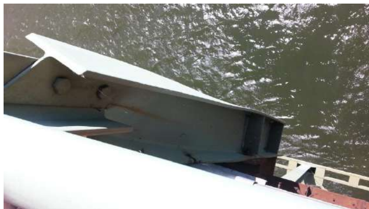
Figure 7. Span 17, distortion limits in post.
