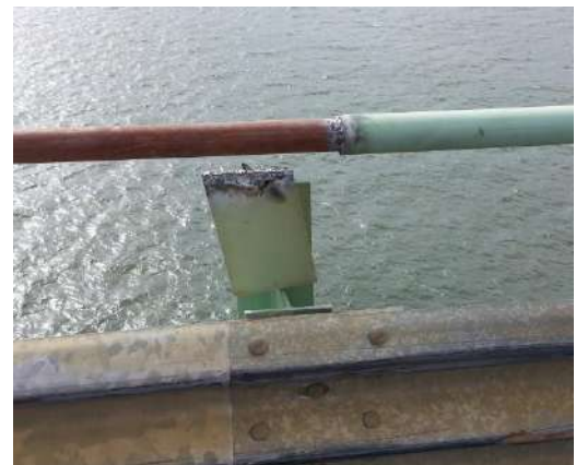
Figure 4. Span 16, P11 severe damage to WT pipe connection.
