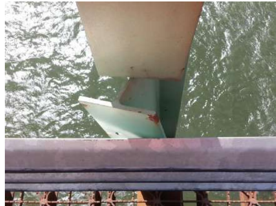
Figure 6. Span 17, P30 significant post deformation
