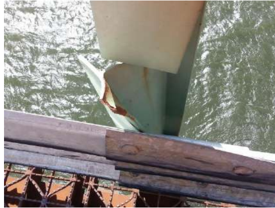
Figure 5. Span 17, P32 significant post deformation
